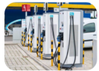
Charging Point Monitoring
